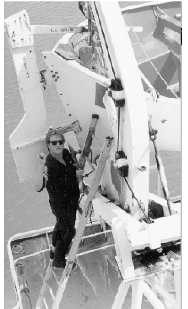
Mike Freng repairing the lifeboat gravity davits for annual inspection. Photo submitted by Dan McDonald.
