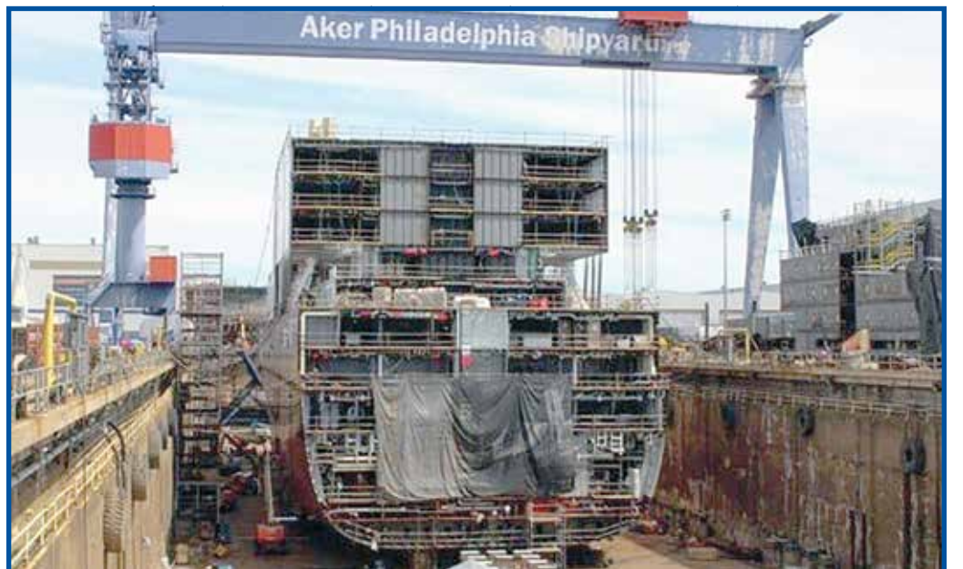
Ship under construction in the drydock of the Philly Yard on the Delaware River, in Philadelphia PA.
